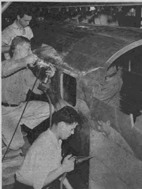
Covering the subject. These sheet-metal workers apply sheet duralumin cover to the metal framework.
