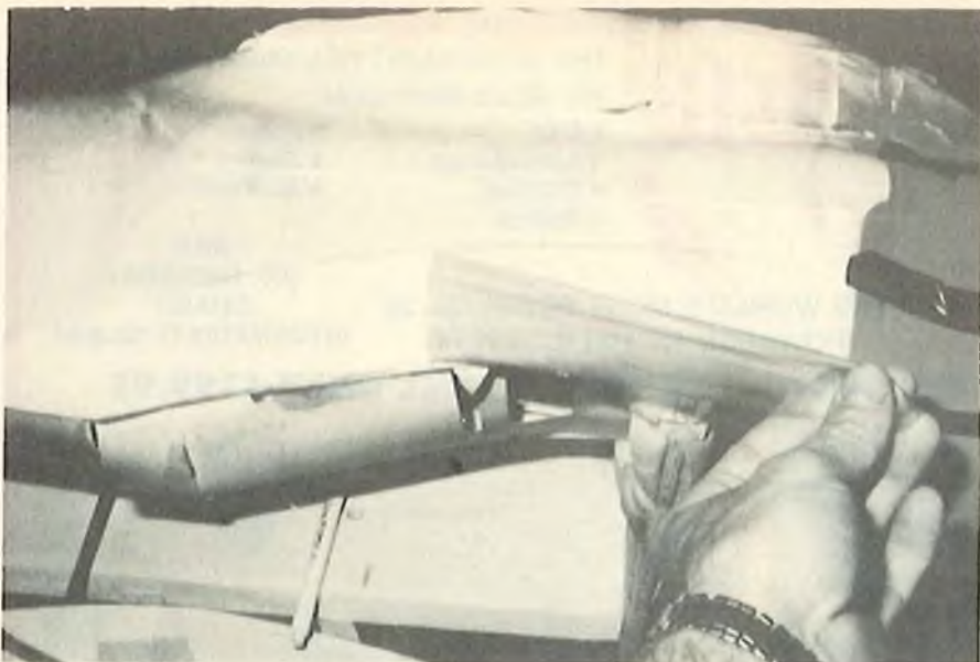
Peeling up LMF. Area to be painted flat black.
