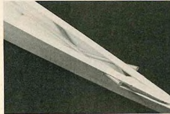
Outer NyRods are installed in fuselage before top sheeting is in place.
