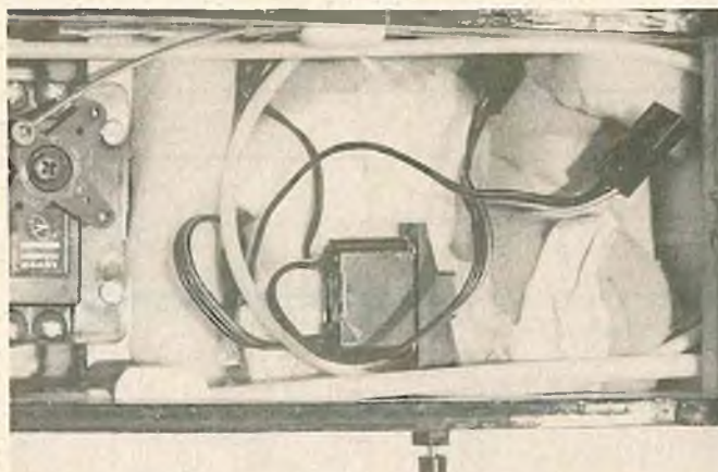
Receiver switch mounted in a Du-Bro switch mount. Makes a neat installation.
