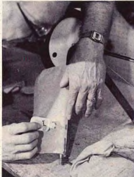
Once pulled tight, seam is glued from top to bottom so that edge of dacron is glued to back of strut.
