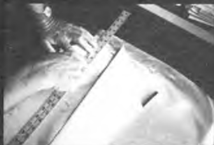
Cutting the glass cloth to fit wing. Allow to completely envelope the wing.
