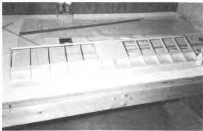
Wing skin cemented to ribs and leading edge. Held in position by pins while upside down on building surface.
