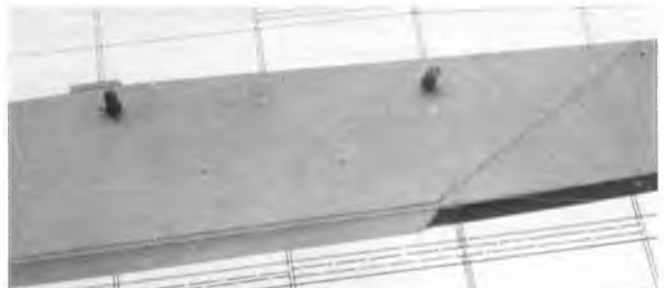
Drill dowel holes. Double check locations — you may have the wrong bay.
