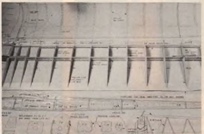
Right wing pinned to assembly board. Shear webs are glued in place.
