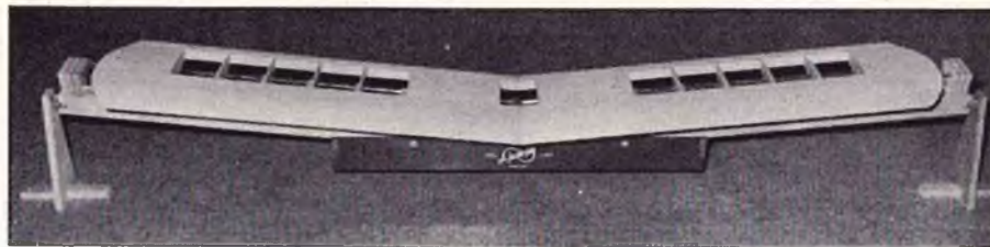
Completed Cherokee wing ready for removal from jig. Only center planking and tips yet to be sheeted.
