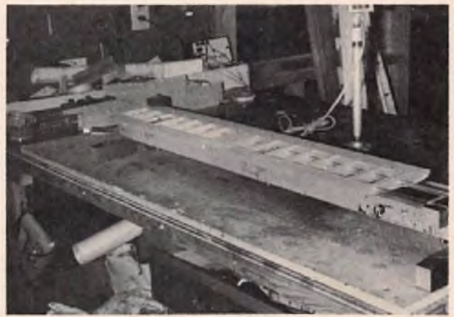
Stab framed & sheeted on top only. Ready to turn over and complete bottom side.
