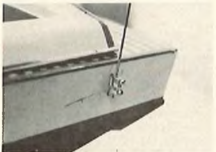
A brass connector from a domino block, silver soldered to a piece of wire which is epoxied to hull. Aerial held in place by BOTH screws.
