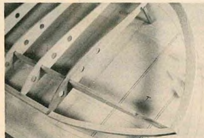
Tip pieces are cut and glued in place, then last tip ribs are installed.
