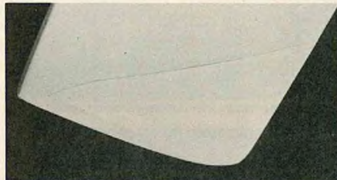
Photo #5b: Patch must be extended to a structural member.
