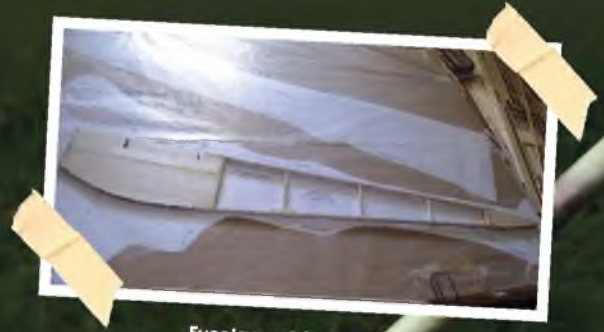
Fuselage side frames are built in the time-honoured manner. Build one over the plan, turn it over and build the other one on top of it.
