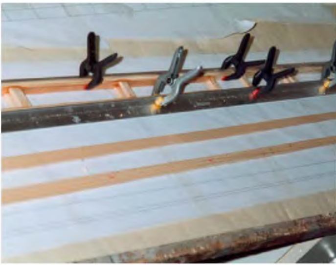
A metal straight-edge is used to ensure that the mainspar is true.
