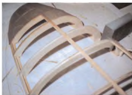
The start of the fuselage surface panelling, with panels covering the forward nose section.
