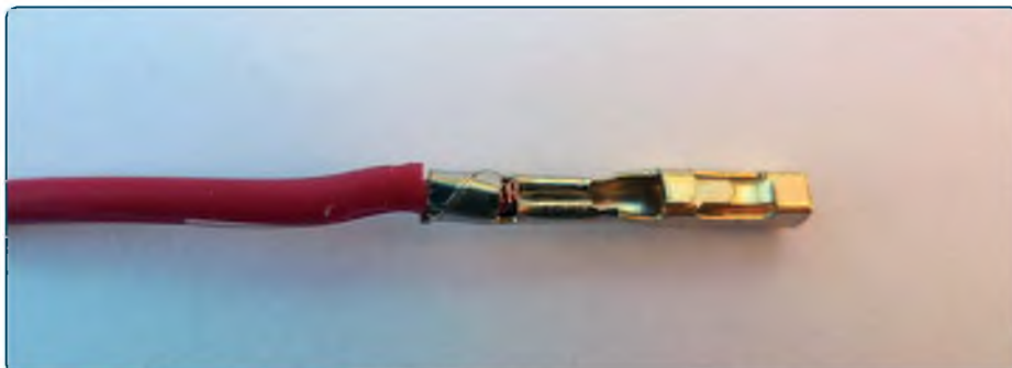
A poor crimp. The wire is not in the correct position so the long outer tangs are not gripping the insulation
