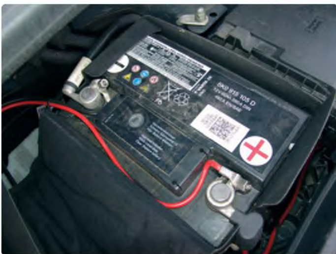
Wire leads are soldered to cable eyelets and screwed directly to both car battery poles
