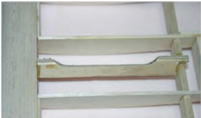
Ply ribs for supporting the strut brackets were fitted in the wing
