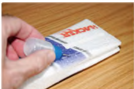
Securing the carbon reinforcing rods using a dropper bottle to get the glue in deep
