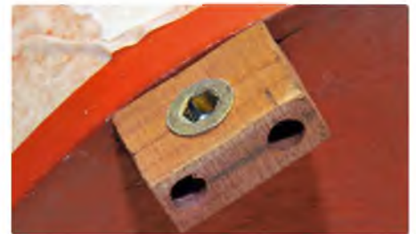
Block mounted to bulkhead
