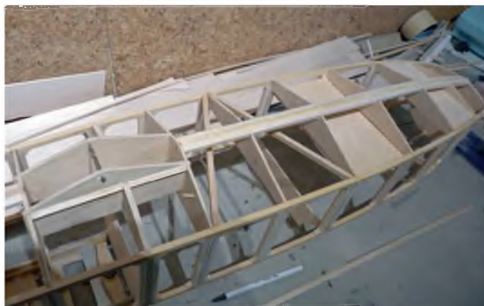
6 mm square spruce diagonals are used to keep the front of the fuselage straight
