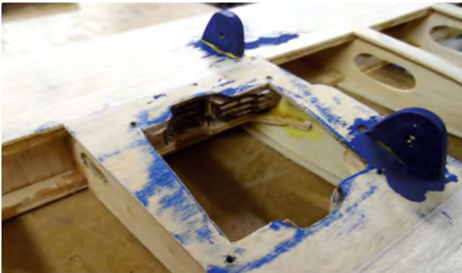
Stripping away the Glosstex revealed a fairly light airframe that was in good condition
