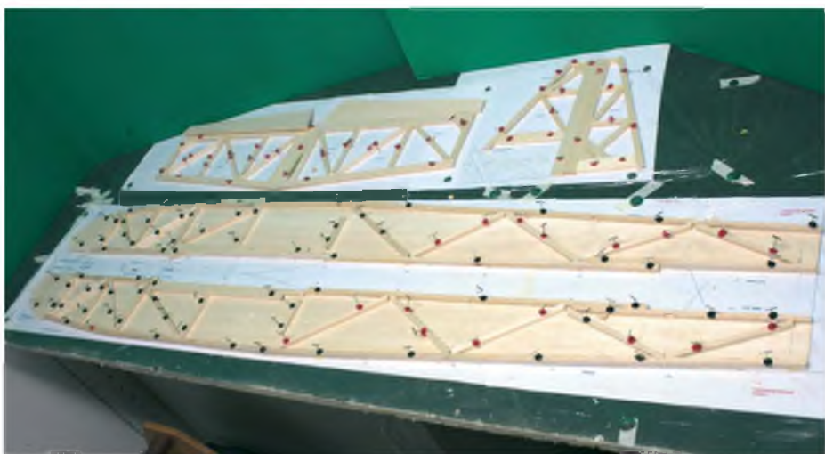
A good way to avoid building two of the same fuselage side is by building both sides at once, top to top or bottom to bottom. Red and black discs on the pins are pin clamps, which spread out the force of the pin and lessen any denting of the wood
