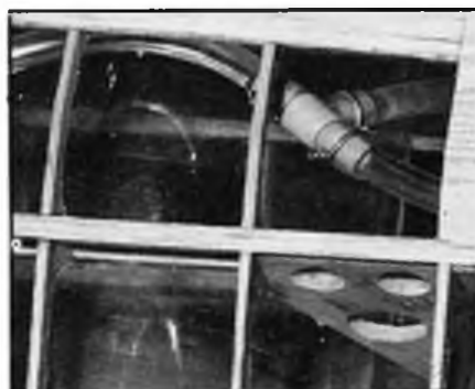
T-piece joining pressure feed from bottle to twin engine pipes.
